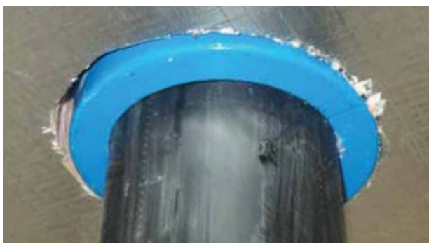
Figure 7 Penetration example - Kingspan Kooltherm® K10 FM G2 Soffit Board installed tight around the fire collar and HDPE service pipe.
